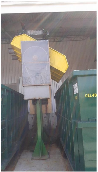
Electro Controls for Deflector
